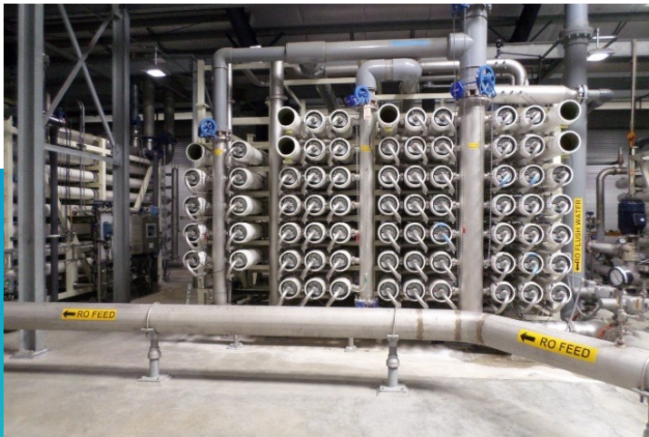
Original RO System
