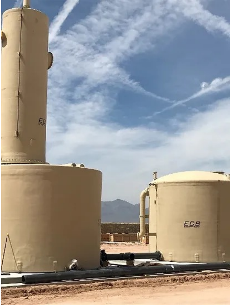
Critical Minerals Corporation Facility in El Paso
