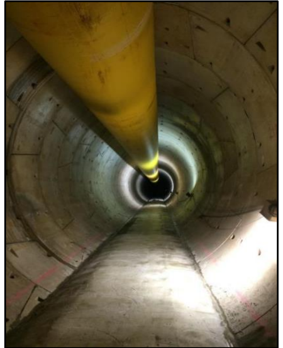
Before Intake No. 3 was put into service
