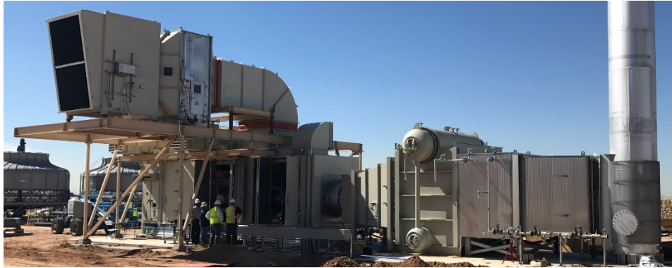
6.5 MW Natural Gas CHP
