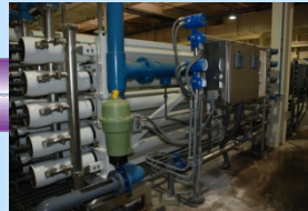
Advanced Water Treatment Plant
