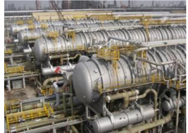
Reliance, India 160,000 m 3 /day MED desalination facility
