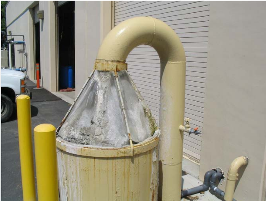
Mineral Deposits on Arlington Desalter Air-Gap Discharge to SARI
